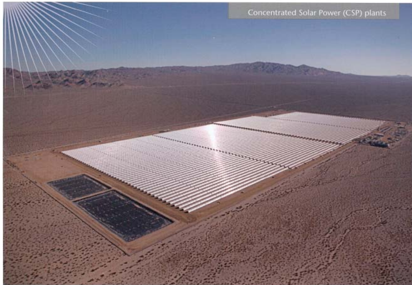
The Concentrated Solar Power (CSP) plant Nevada Solar I was installed close to Boulder City, USA, in June 2007. It has an output of 64 MW. With an area of 7.4 million m 2 it is as large as 212 football fields.
