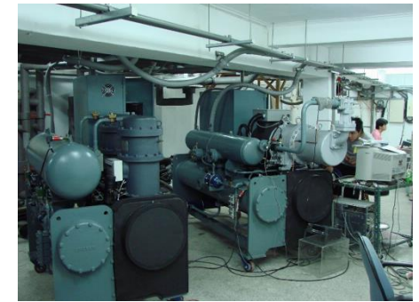
高效率變頻製冷主機開發 High-efficiency refrigeration system with VSD control
